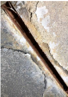
Muffel offene Fugen
